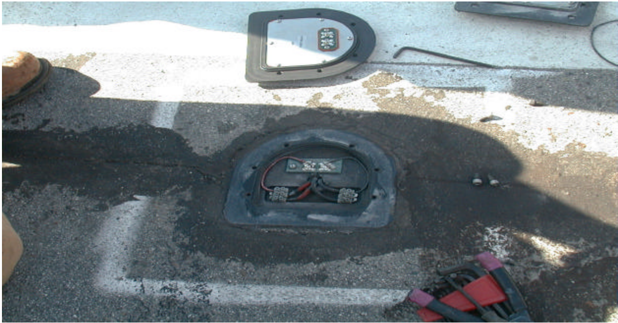
Figure 6: Embedded pavement flashing light system housing fixture
